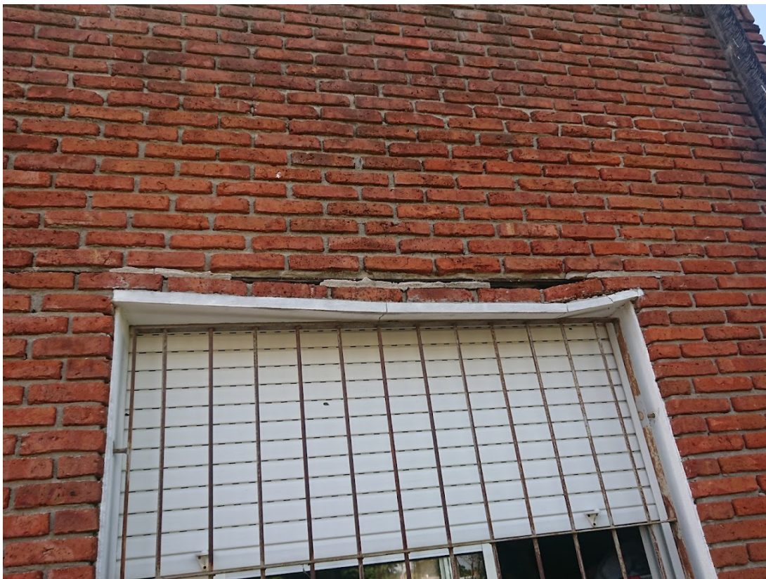
Dinteles a reparar (total 4)
