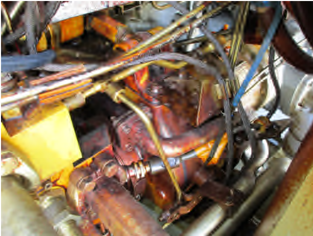
Picture 3: Discoloration on lube & scavenge pump
